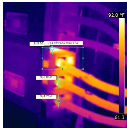
Fig 5 – Temperature Differences between Three Sockets
